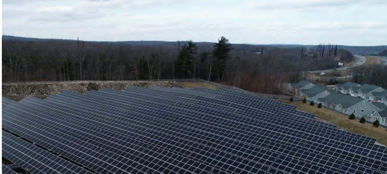
JOHNSTON-SCITUATE SOLAR: The Johnston-Scituate solar project, a 4.675 MW solar project on 17 acres along Scituate Avenue in Johnston, has been operational since 2021. (Photo courtesy Green Development)
